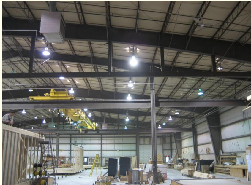
Figure 8: Industry Environment, using a Metal Halide bay lighting system at 4000k (Huntington Homes, 2016)
